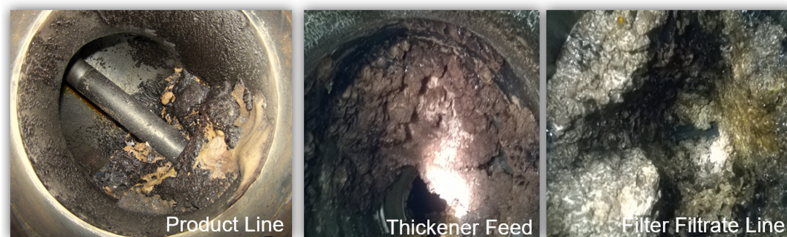
Figure 8. Oxalate scale in pipework.
